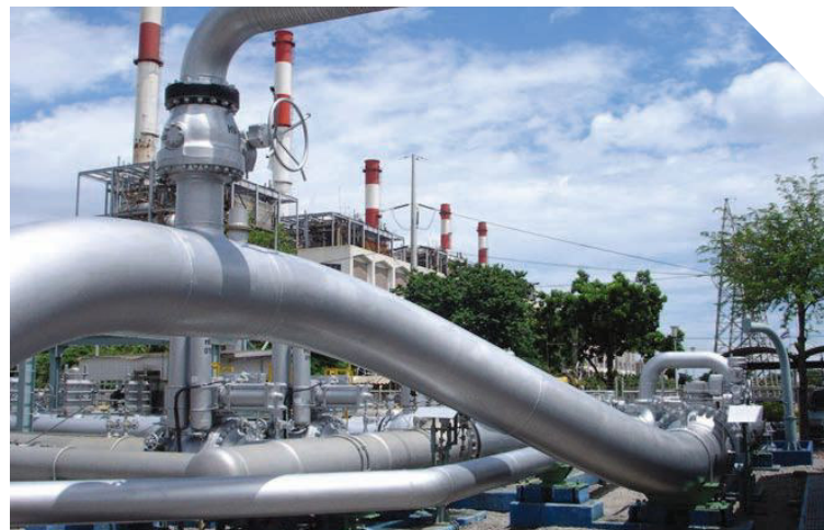
PTT's engineering team designed a gas transmission pipeline Block Valve Station that controls and measures the supply of natural gas to South Bangkok Power Plant.
